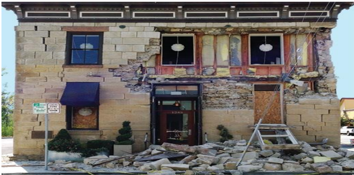
Figure 7 – Damaged old masonry building built in 1875, during the earthquake in South Napa, California, in 2014.
