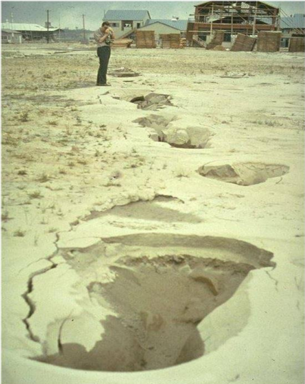
Figure 13 – Liquefaction of sand base as a result of a longitudinal seismic wave in Kobe, Japan.
