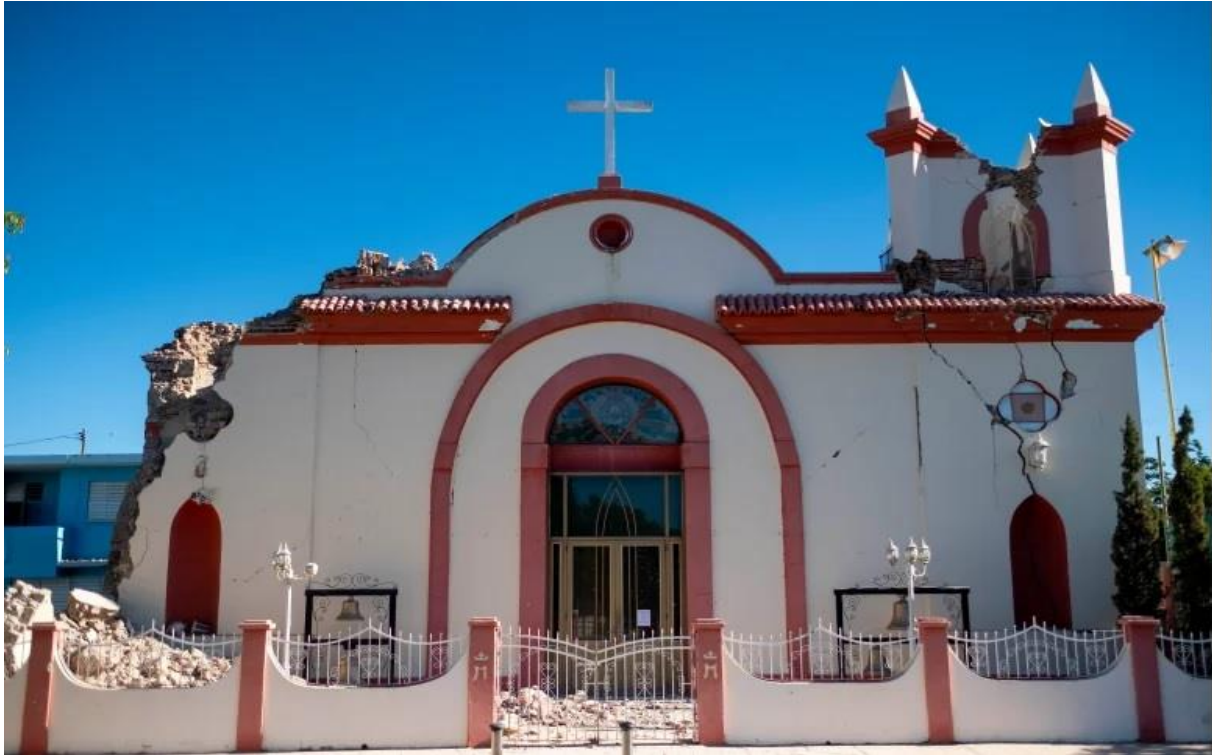
Figure 9 – Partially collapsed old Inmaculada Concepcion church built in 1841, after the 2020 earthquake on the island of Guayanilla, Puerto Rico.
