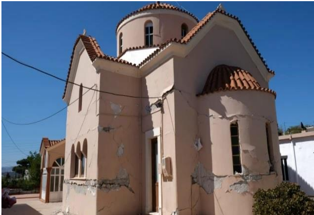
Figure 11 – Damaged Greek Orthodox church on the island of Crete in Greece as a result of the Arkalochori earthquake in 2021.
